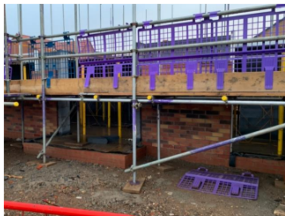
Figure 2. Example of compromised access due to 1st lift scaffold being erected prior to Access Platform Decking system installation
