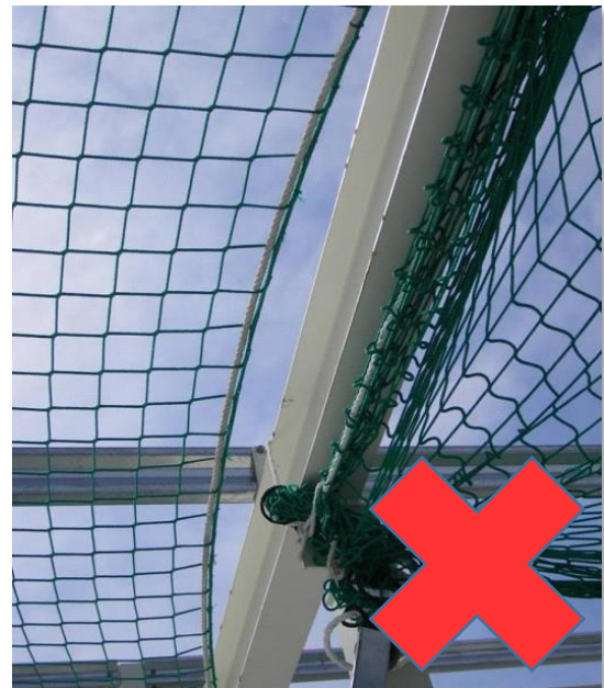
Figure 2. Safety Nets installed with excessive gaps
